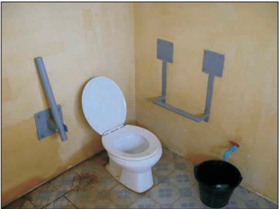
Photo 7. Adaptation of grab bars in accessible toilet
