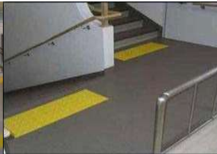
Figure 37- Warning blocks at landings
