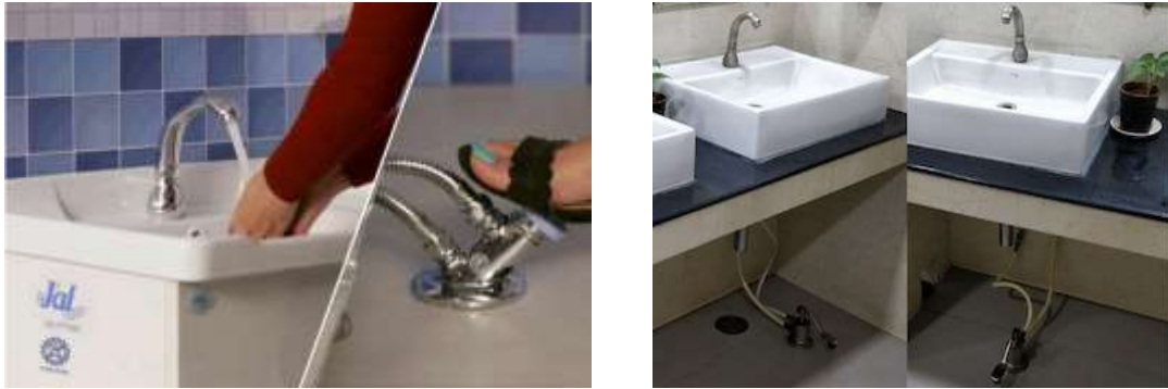
Figure 61- Foot operating tap
